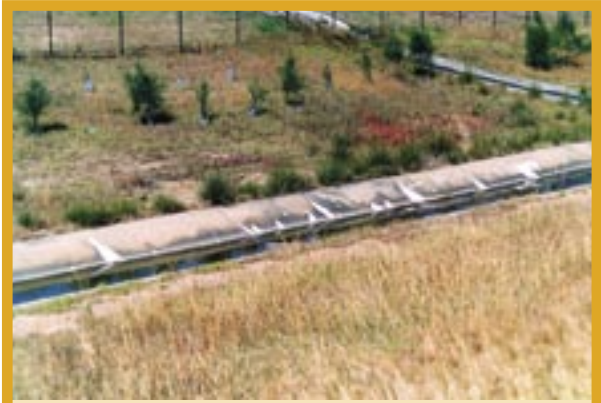
Salinity indicator plants, salt crystals, groundwater seepage and poor soil structure are evident in this stormwater easement through an industrial area. Tree planting will help lessen the impacts of salinity processes while providing other benefits such as habitat.
