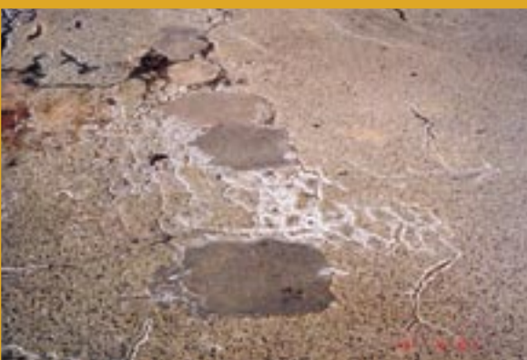
Water affects the stability of the layers that support a road, while the concentration of salts through evaporative processes physically and chemically react with the construction materials.
