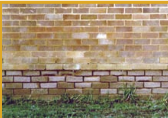
Salt and water are entering the brickwork from the ground. Evaporation results in the formation of salt crystals. These exert pressure on the bricks so that grain by grain the brick crumbles.
