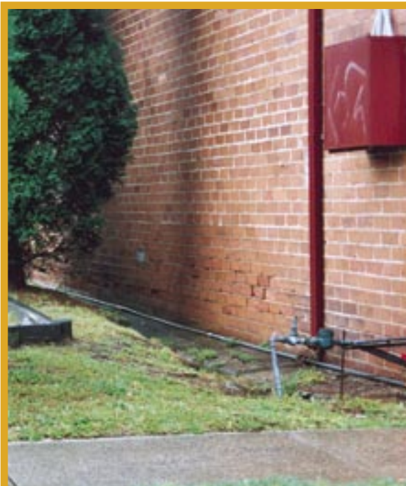
Water and salt are impacting on the mortar on this wall. Discharge of stormwater directly at the base of the wall is exacerbating the effects of local conditions.
