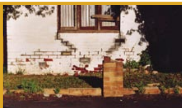
Salt and water have affected the paintwork and mortar on this property. Exposure class bricks and mortar are more resistant to the impacts of salinity.
