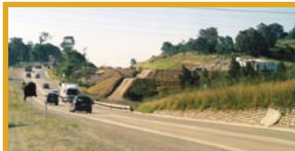
This photo illustrates the extensive earthworks that are sometimes undertaken for urban development. This may expose saline or sodic subsoils, result in these soils being dumped in other locations and may also interfere with natural surface and subsurface drainage patterns.
