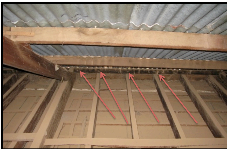
Figure 3.13 above: Photograph showing small circular vent holes in the eaves line located roughly at the end of each ceiling joist. Location indicated by the red arrows Photograph by Tuck, June 2013
