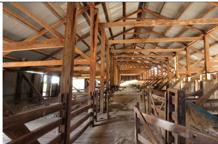
Figure 3.32 An interior view of the Dunlop Shearing Shed. Photographs by Sheppard April 2013.
