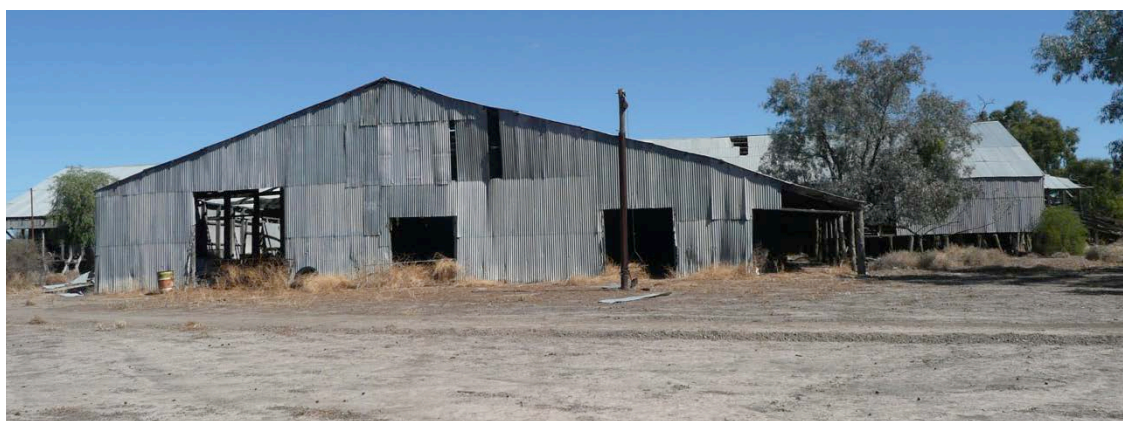
Figure 3.31 East and west elevations of the Dunlop Shearing Shed. Photographs by Sheppard, April 2013.
