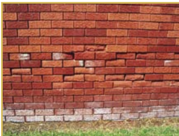
Crumbling bricks and mortar, the presence of rising damp and salt crystals are all indicators that suggest this building is affected by salinity. Photo: DIPNR
