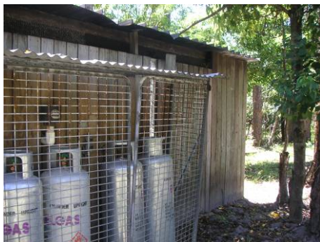
Picture 27 – Generator shed
