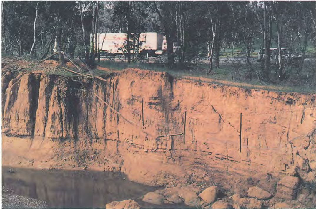
Plate 5: Undercutting and collapse causing creek to trespass onto Hume Highway easement. Photo Mullengandra Creek catchment.
