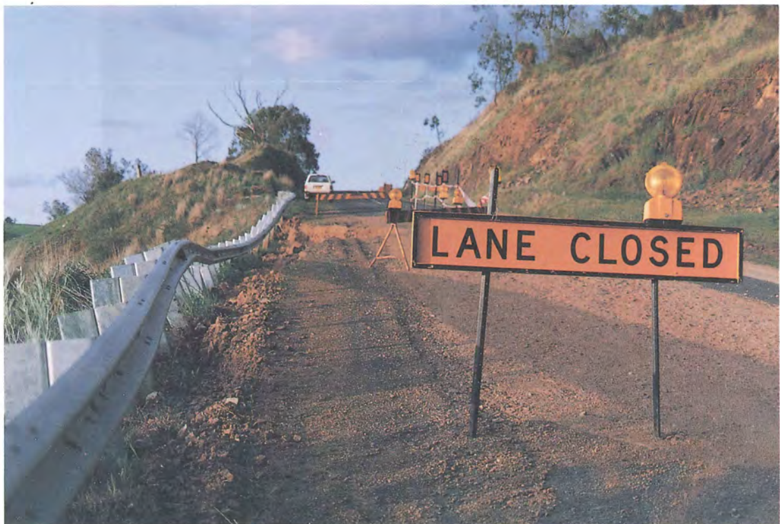
Plate 14: Slumping on unstable slopes in Basalt areas can result in costly damage. Photo Tumbarumba-Tooma Road, Tumbarumba Creek catchment.
