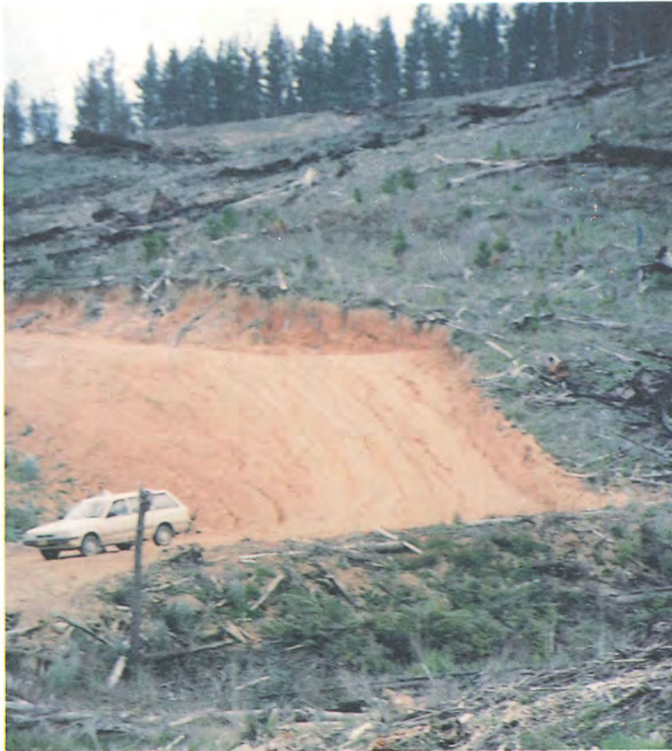
Plate 15: Erosion associated with roadworks required for pine harvesting and re-establishment.
