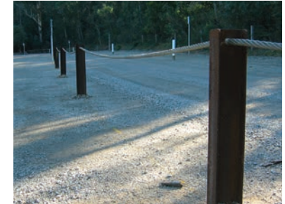
Steel post and cable barriers
