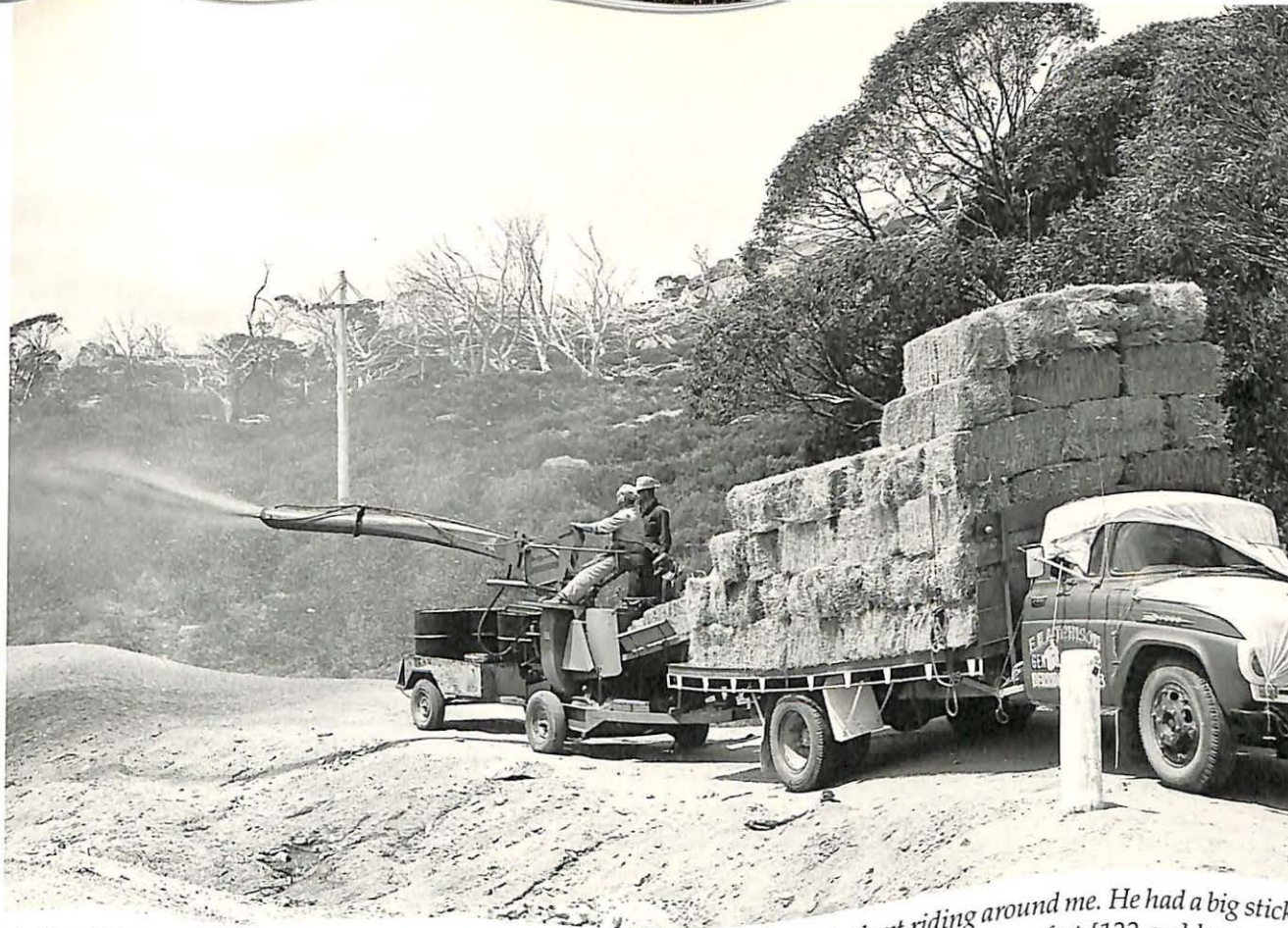
The Finn Mulcher in operation along the Guthega Link Road. It sprayed grass seed mixed with chaff and bitumen to stabilise soil on reshaped areas along roadside batters to prevent them eroding.
