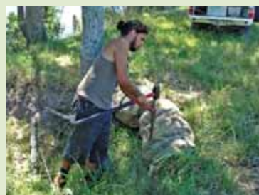
The eco-logs are secured using wooden stakes and shaped into arcs to create a pooling effect which then overflows to the next pool
