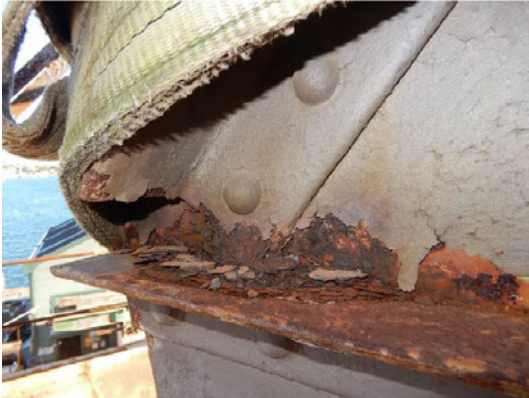
Figure 33: Looking along the jib when the crane was last climbed by an engineer showing extensive corrosion and paint loss. (Arcadis, July 2021)
