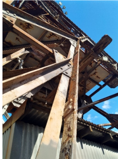
Figure 30: Looking up a tower leg, showing considerable corrosion. (TTW, June 2022).
