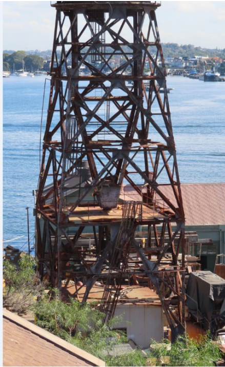
Figure 216: The crane tower, with the slew ring at the top. (R Newton/NPWS, 2024)
