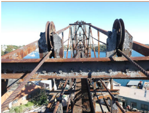
Figure 31: Looking along the jib when the crane was last climbed by an engineer showing extensive corrosion and paint loss. (Arcadis, July 2021)
