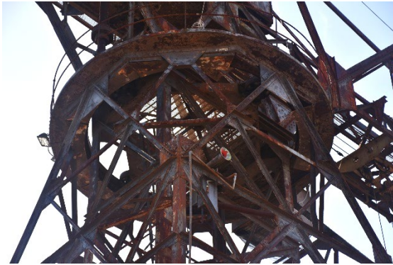
Figure 135: Looking up to the slew ring under the jib showing extensive corrosion. (TTW June 2022)
