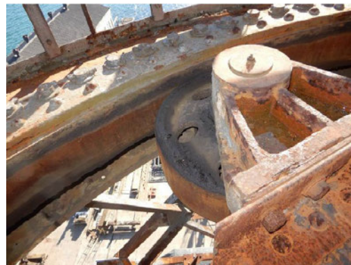
Figure 318: Looking along the jib when the crane was last climbed by an engineer showing extensive corrosion and paint loss. (Arcadis, July 2021)
