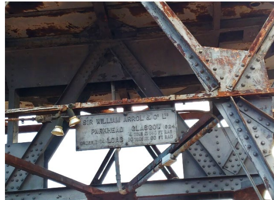
Figure 168: The manufacturer's plaque bolted to the tower. (TTW, June 2022).
