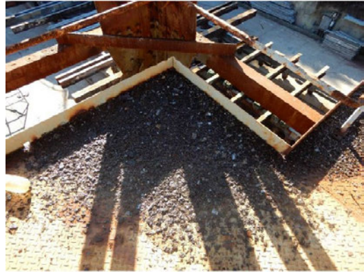
Figure 194: Looking onto the Level 1 Platform when the crane was last climbed by an engineer showing extensive corrosion. (Arcadis, July 2021)
