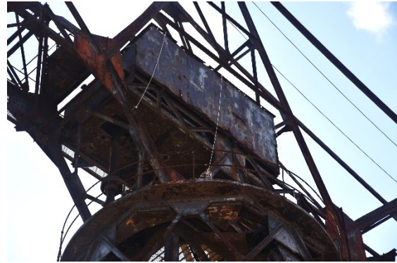
Figure 146: Looking up to the underside of the motor room showing extensive corrosion. (TTW June 2022)
