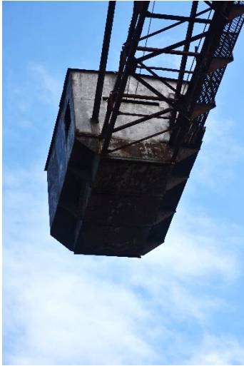
Figure 179: Looking up to the underside of the winch room at the short end of the jib showing extensive corrosion. (TTW, June 2022).
