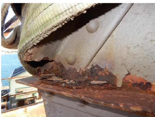
Figure 46. Looking at the bottom of the rotating mechanism when the crane was last climbed by an engineer showing extensive corrosion (Arcadis July 2021)
