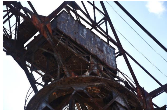
Figure 39. Looking up to the underside of the motor room showing extensive corrosion. (TTW, June 2022)
