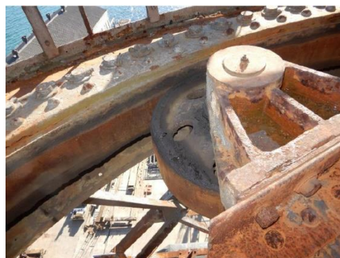
Figure 436. Looking at the slew ring mechanism when the crane was last climbed by an engineer showing corrosion. (Arcadis, July 2021)
