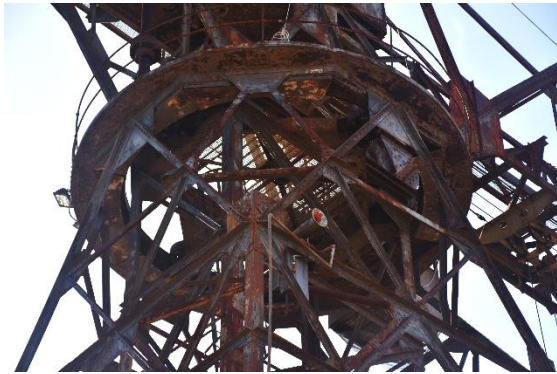
Figure 3831. Looking up to the slew ring under the jib showing extensive corrosion. (TTW, June 2022)
