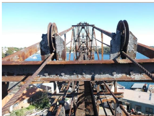
Figure 44. Looking along the jib when the crane was last climbed by an engineer showing extensive corrosion and paint loss (Arcadis, July 2021)
