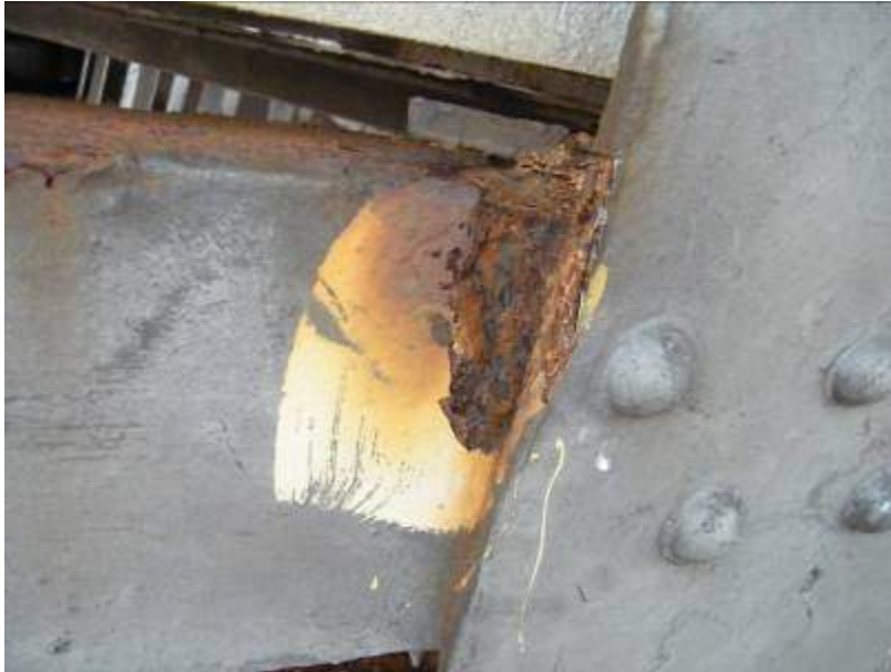
Figure 3 Typical severe corrosion
