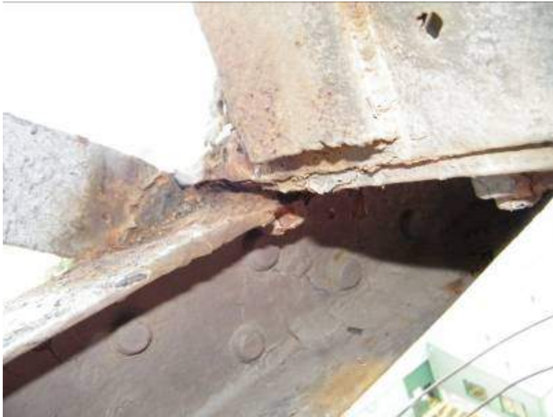
Figure 4 Main structural members reduced in thickness by over 50% by corrosion damage
