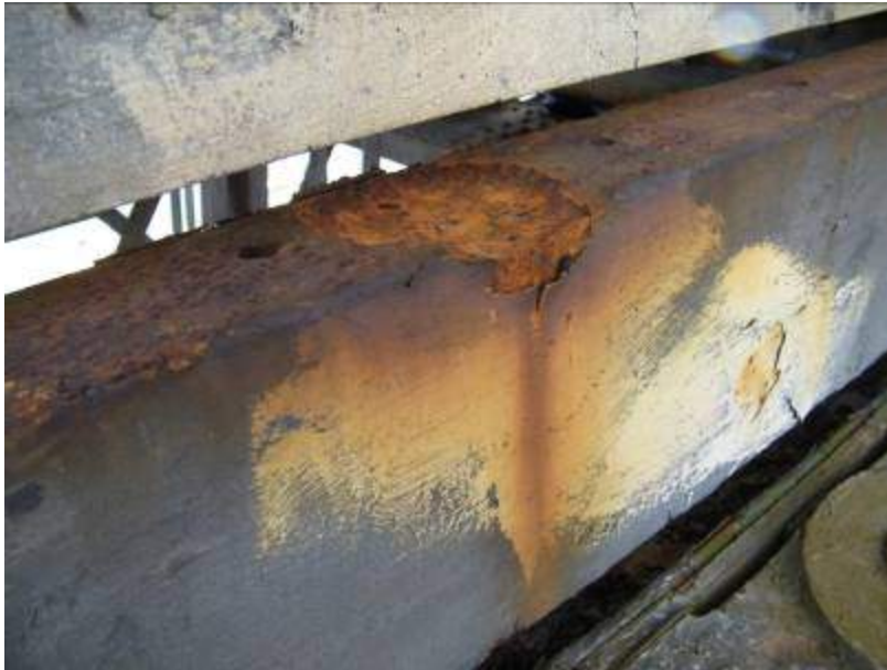
Figure 16 Corrosion in main boom structure
