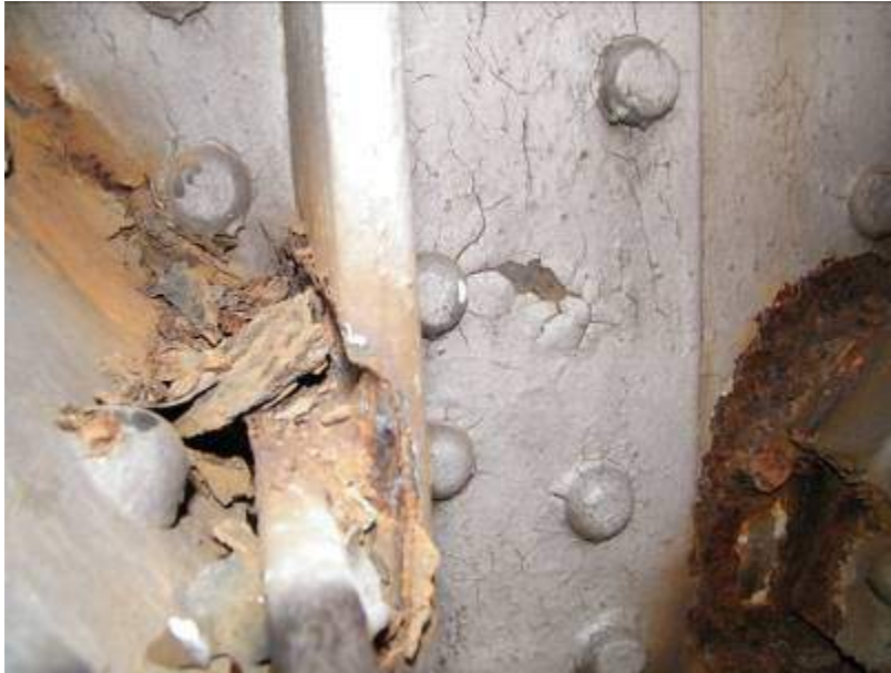
Figure 15 Severe corrosion in main frame plates
