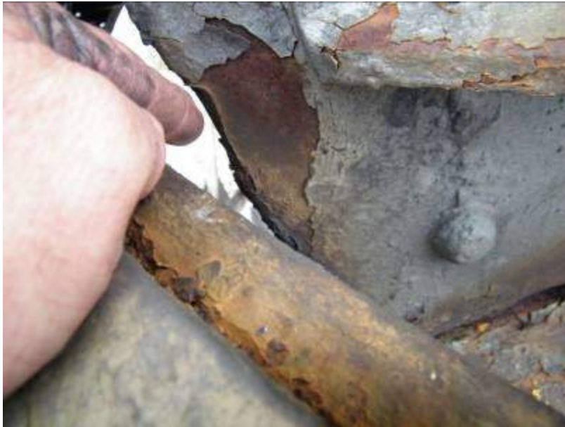
Figure 10 Evidence of impact between frame and slew ring
