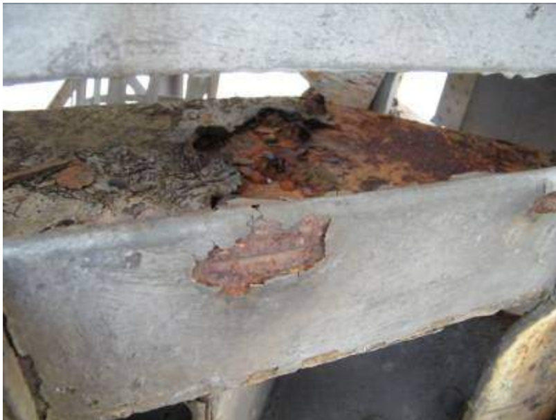
Figure 2 Typical Severe Corrosion - Rivet heads completely corroded away
