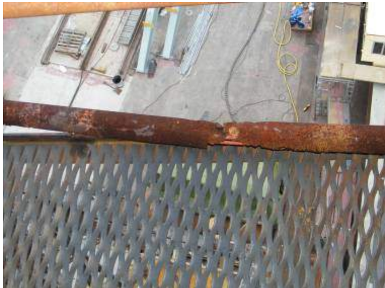
Figure 14 Severely corroded electrical conduit
