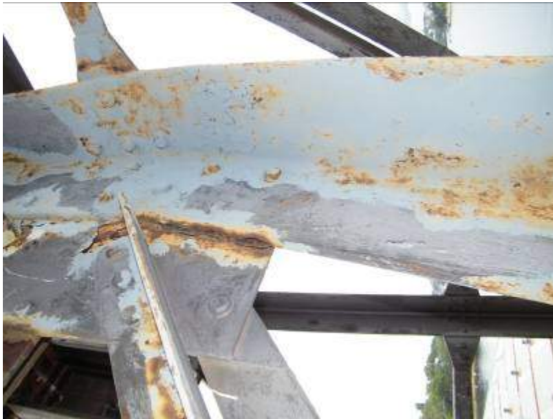
Figure 13 Corrosion between plates
