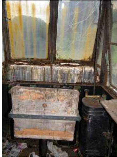
Figure 7 Damaged window in main control cabin
