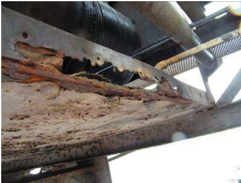
Figure 6 Excessive Corrosion on racking winch mount
