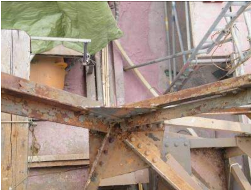
Figure 12 Typical Flaking Paint
