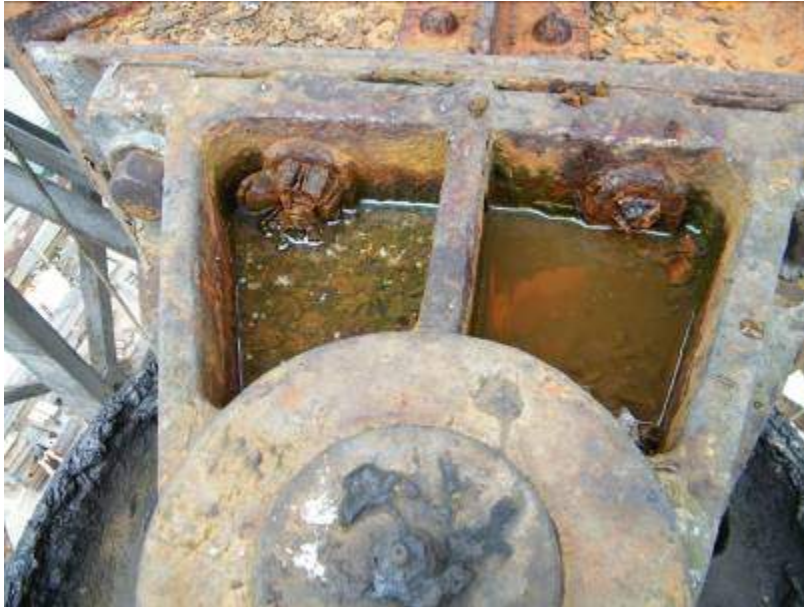
Figure 9 Bolt heads removed by corrosion damage on slew rollers
