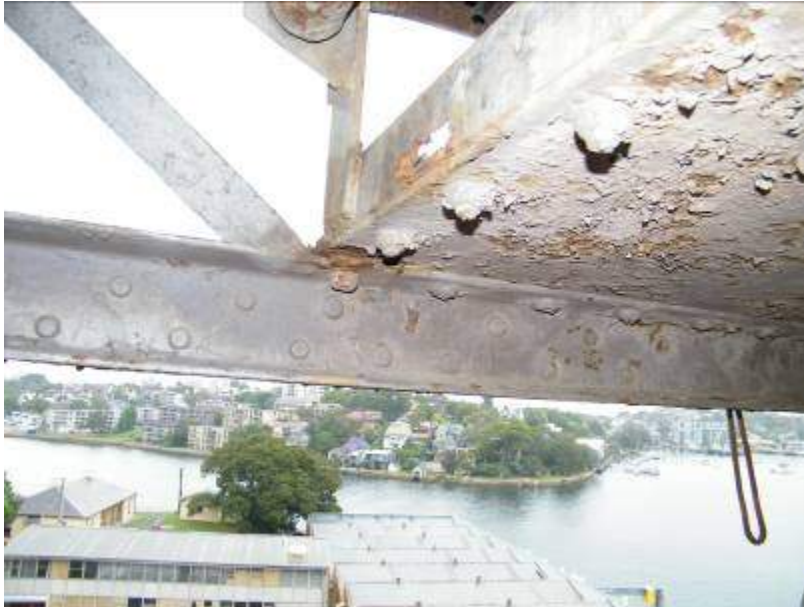
Figure 5 Excessive corrosion on racking winch mount
