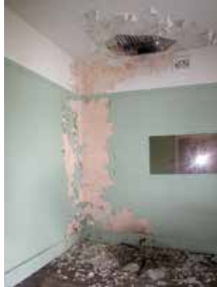
Bedroom with damaged plaster, Residential Cottage No. 3
