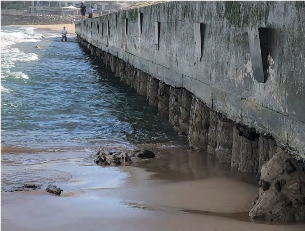
Figure 8-9: Low beach level and exposed contiguous pile face, dated 4 November 2020
