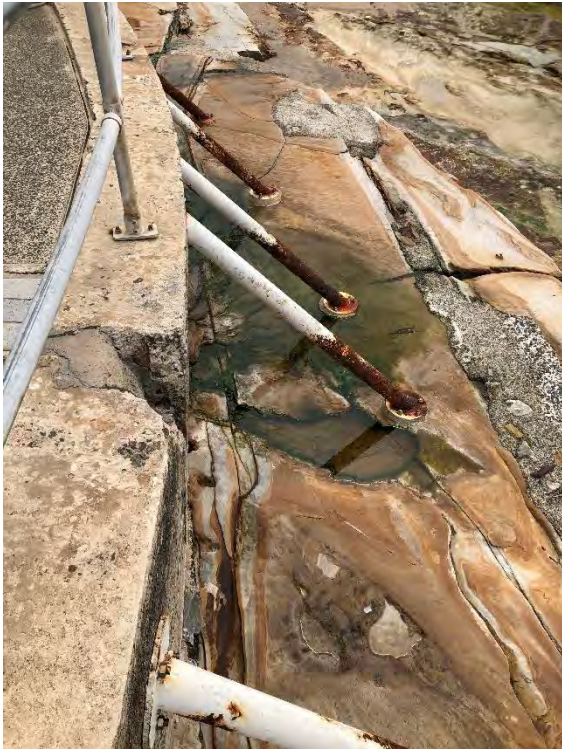
Figure 3-9: Displaced section of The Esplanade stabilised through use of props
