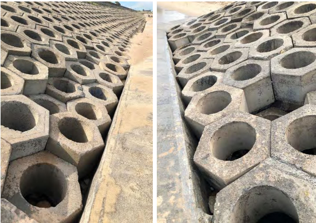
Figure 8-10: Subsided Seabee units (left) and Seabee units spanning over large cavities where individual units have dropped (right)
