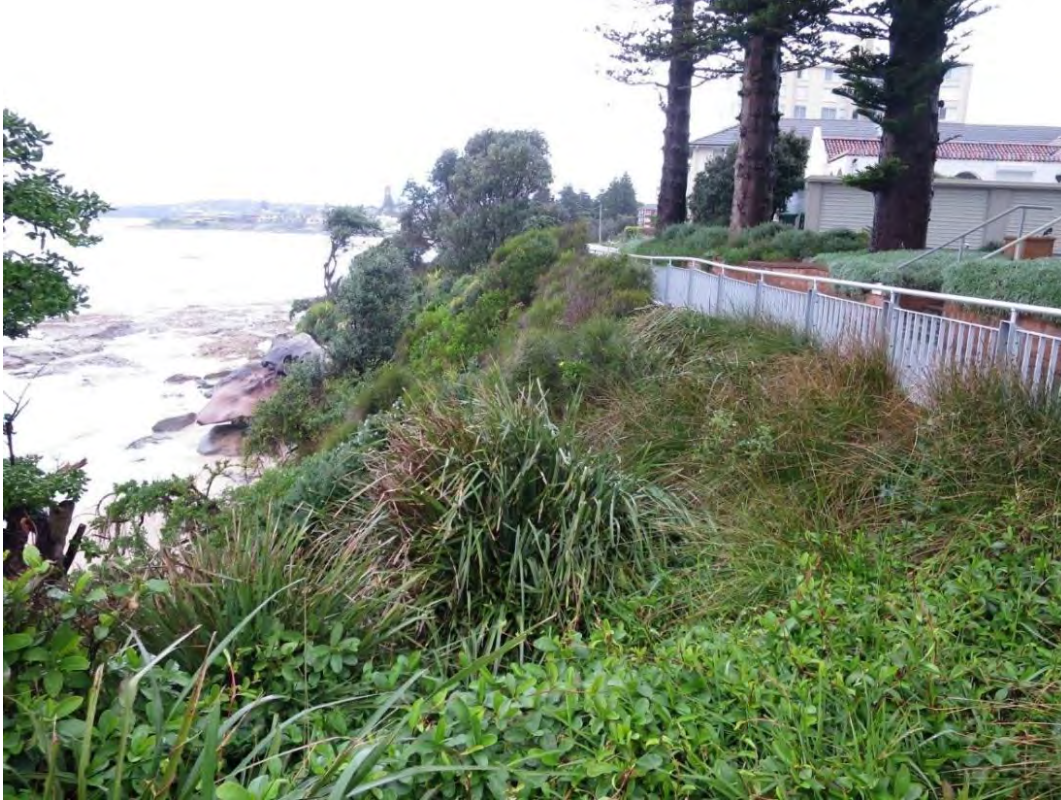
Figure 8-3: Foreshore soil slopes above the crest of the cliff line between 25 Elizabeth Place and 12 Arthur Avenue (i)
