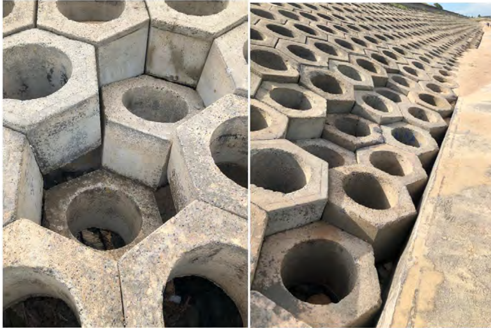
Figure 7-4: Undermined Seabee units at Prince Street Seawall, 2020
