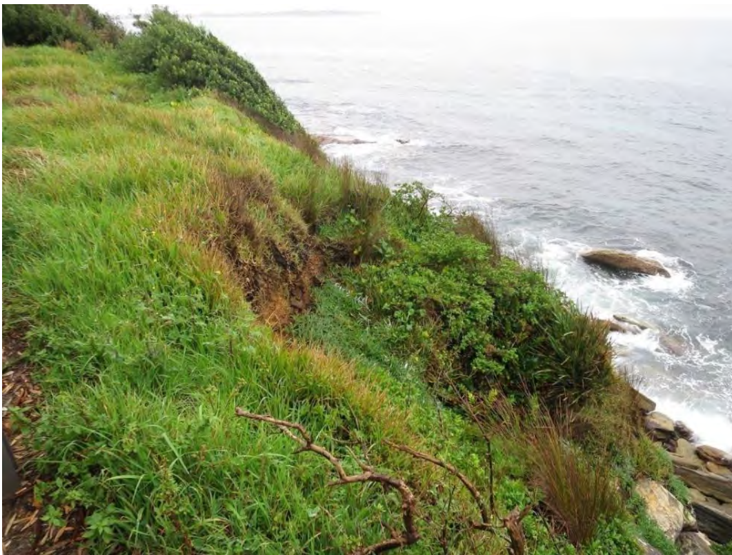
Figure 8-4: Foreshore soil slopes above the crest of the cliff line between 25 Elizabeth Place and 12 Arthur Avenue (ii)
