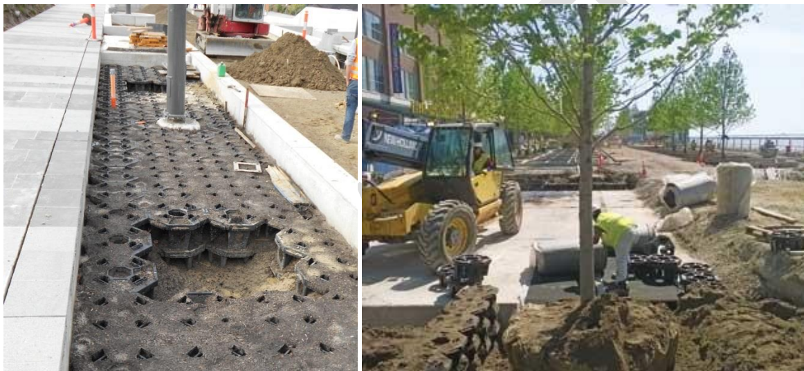
Figures 5.52 and 5.53. StrataCell in City Street, Dandenong (left), ready for tree planting, and in South Dock on Navy Pier, Chicago, US (right). Sources: Maslog-Levis (2012) (left); Landscape Online (n.d.) (right).
