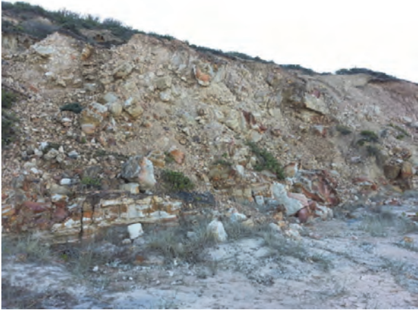
Photograph 9: Ongoing spalling and rockfall from old fill platform at Middle Camp Beach, Catherine Hill Bay, photographed 2015.
