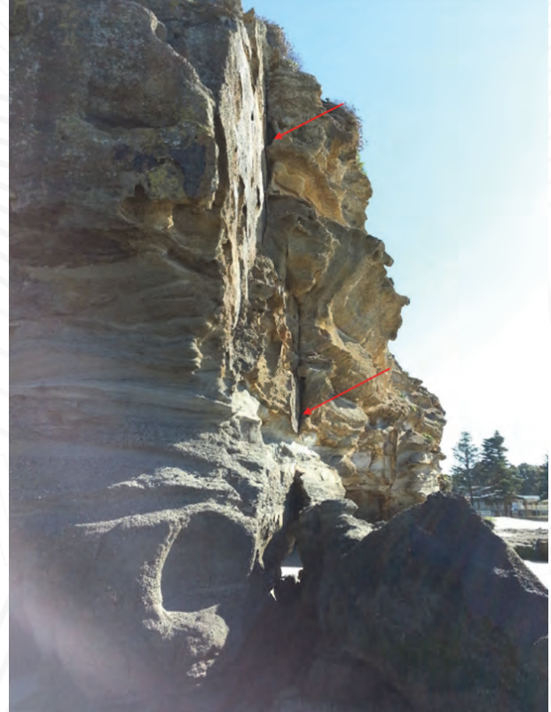
Photograph 7: Potential cliff instability at southern Caves Beach with red arrows showing open joint, photographed 2015.
