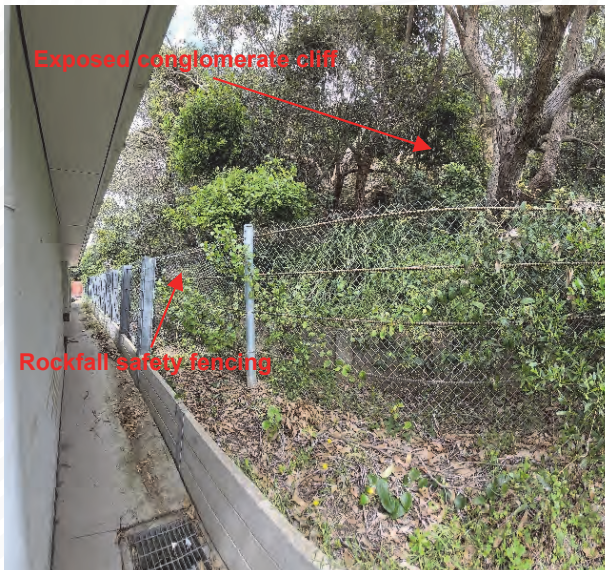
Photograph 6: Caves Beach picnic area, exposed conglomerate with rockfall protection from bushland and safety fencing, photographed January 2021.
