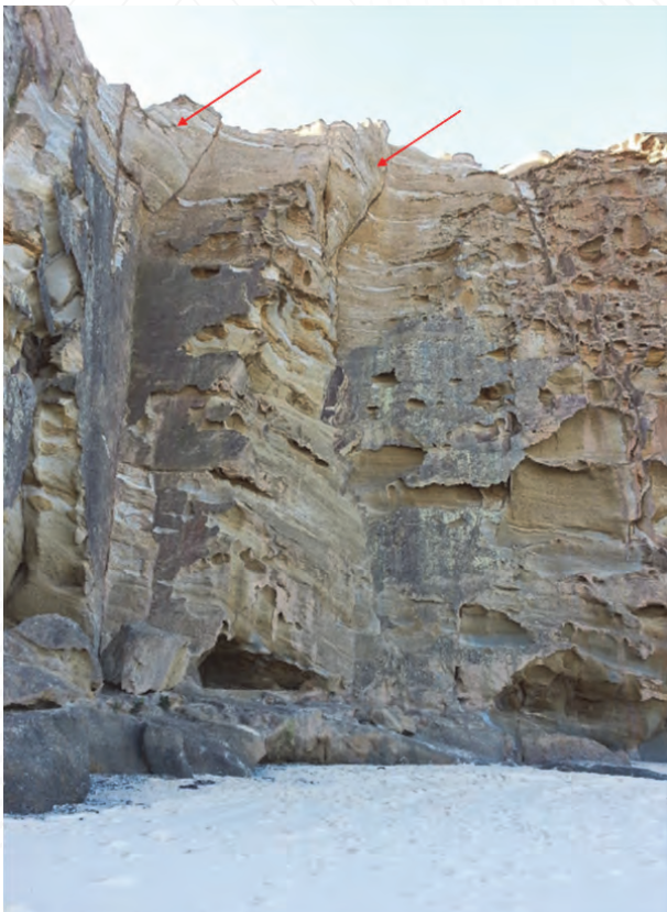
Photograph 1: Insipient failure of rock wedges at southern end of Redhead Bluff, photographed 2015.
