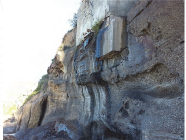
Photograph 11: Old coal pier footings undermined, Catherine Hill Bay, photographed 2015.
