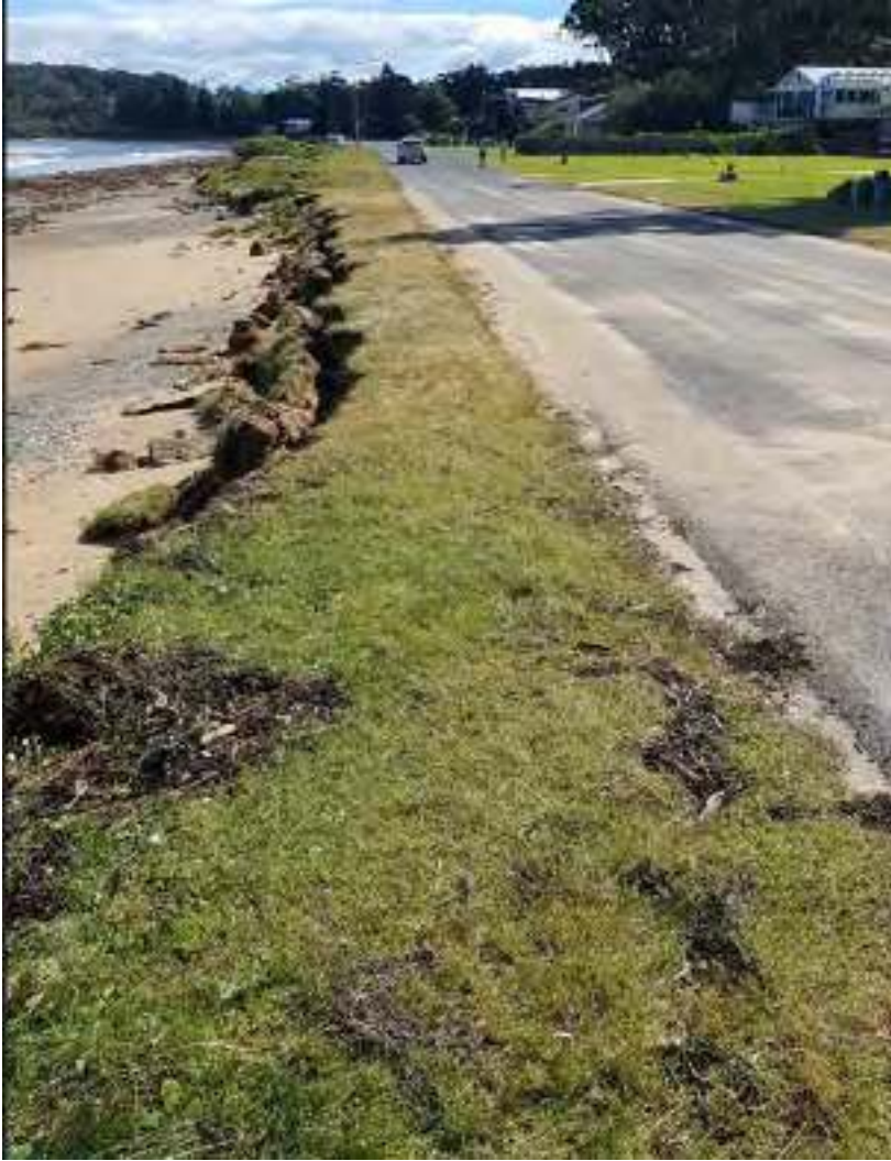
Overtopping of Bay Road, Long Beach, 4 th April 2022 (Mr Cameron Whiting ESC)
