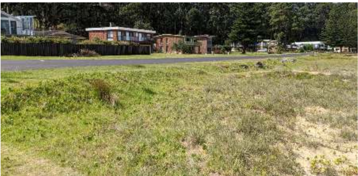
Existing Revetment Structure East of Fauna Ave, Long Beach, 16 March 2021 (Baird Site Visit)
