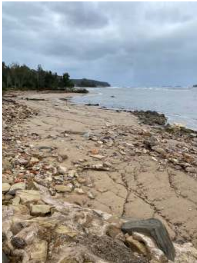
Debris strewn across the beach from the dilapidated seawall, Wharf Road, 4 th April 2022 (Mr Cameron Whiting, ESC)
