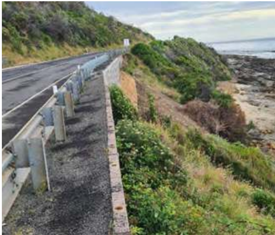
Figure 5 Example of Reinforced concrete wall for stabilisation of a section of the Great Ocean Road, Vic
